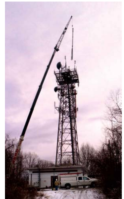
The 40 foot mast on which WDFH's new antenna would be mounted is captured here just moments before being secured to the top of the 125 foot hilltop tower in Mount Pleasant, New York. [January 6, 2009] The antenna installation was completed on January 19 and the new signal went on the air at half power on January 24. The signal went to full power in early February.
